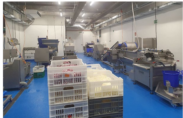
The newly constructed processing center is equipped with several KRONEN processing lines and individual machines
